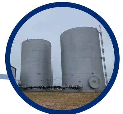
Step 3: Storage Tank
