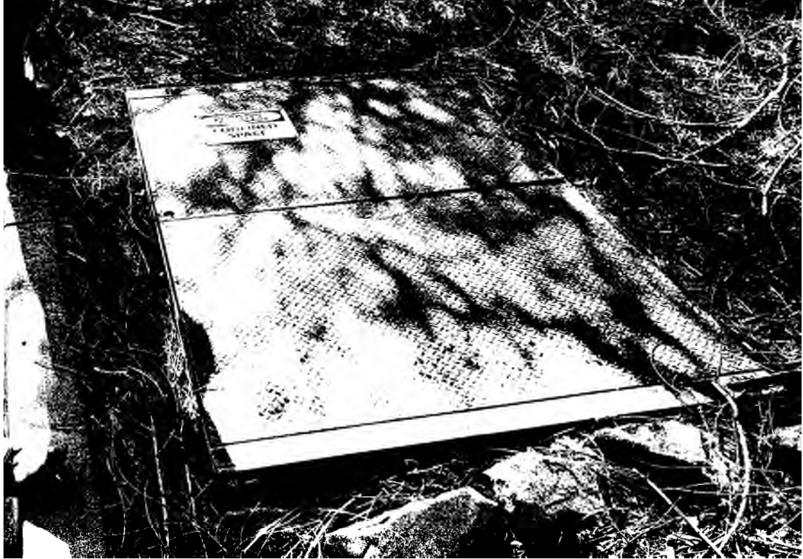
Access to Pressure Reducing Vault on Waxwing Drive
