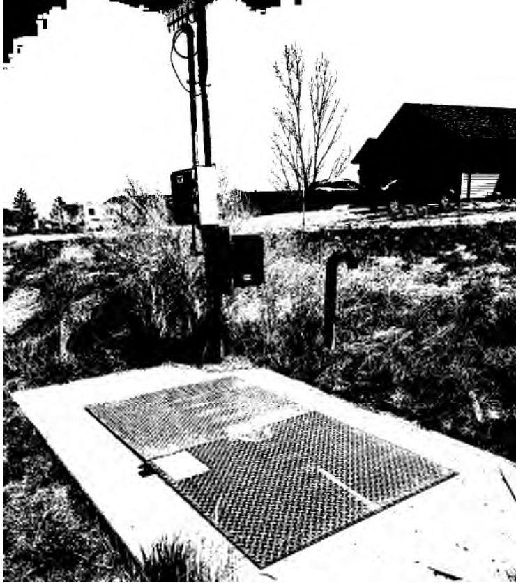
Tract 400 – Oakmont PRV (located at Oakmont and Silver Oak Drives)
