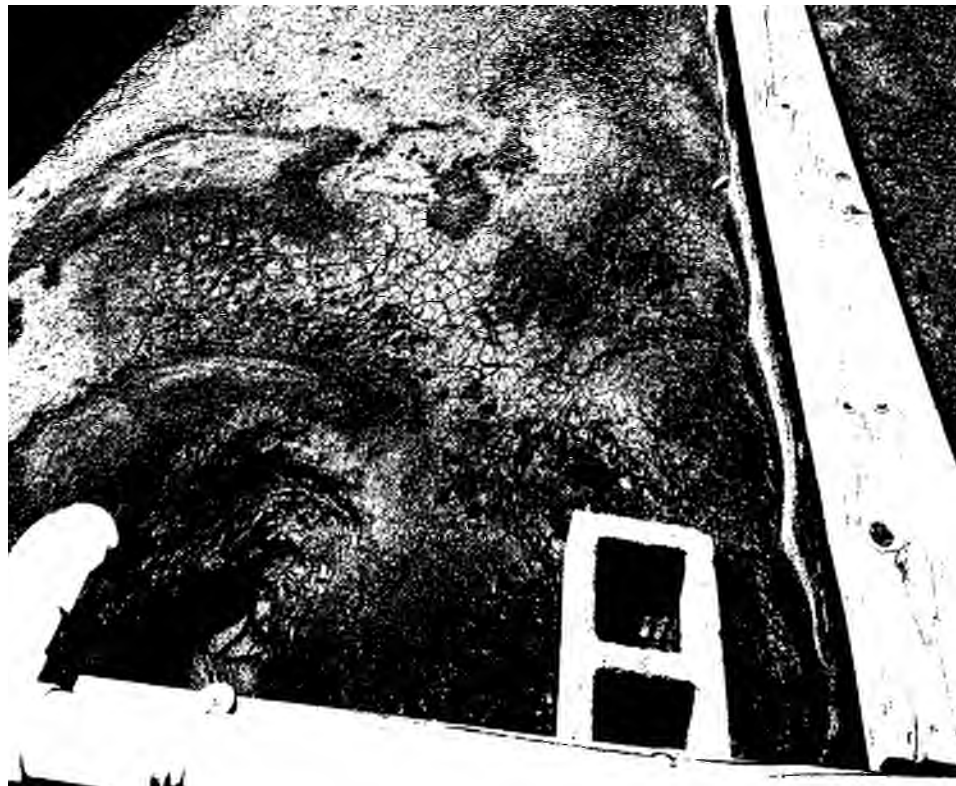
Well #1 Arsenic Treatment Sludge Drying Beds
