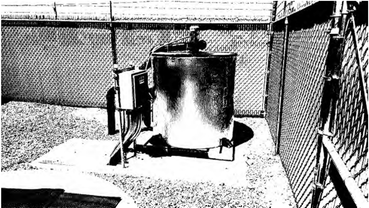
Lift Station #3 Media Order System
