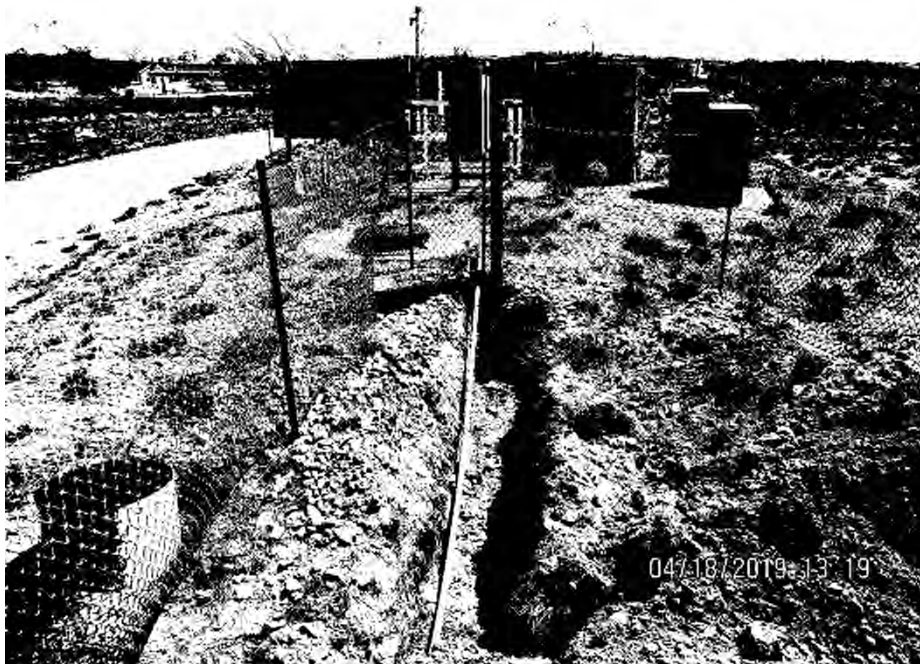
Figure 2: Line to new Ultra Sonic Flow Meter
