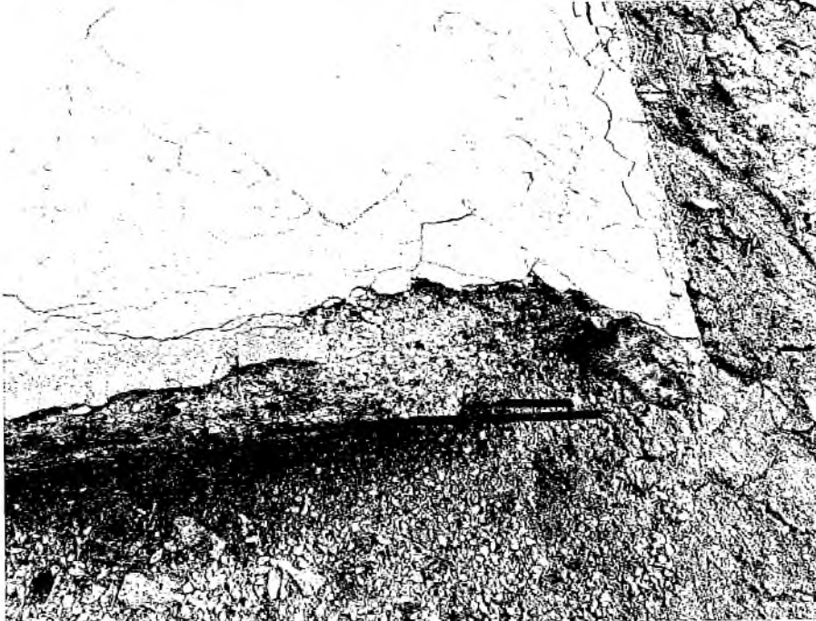
Photograph 5. Deteriorated concrete and corroded reinforcing steel at the northwest corner.
