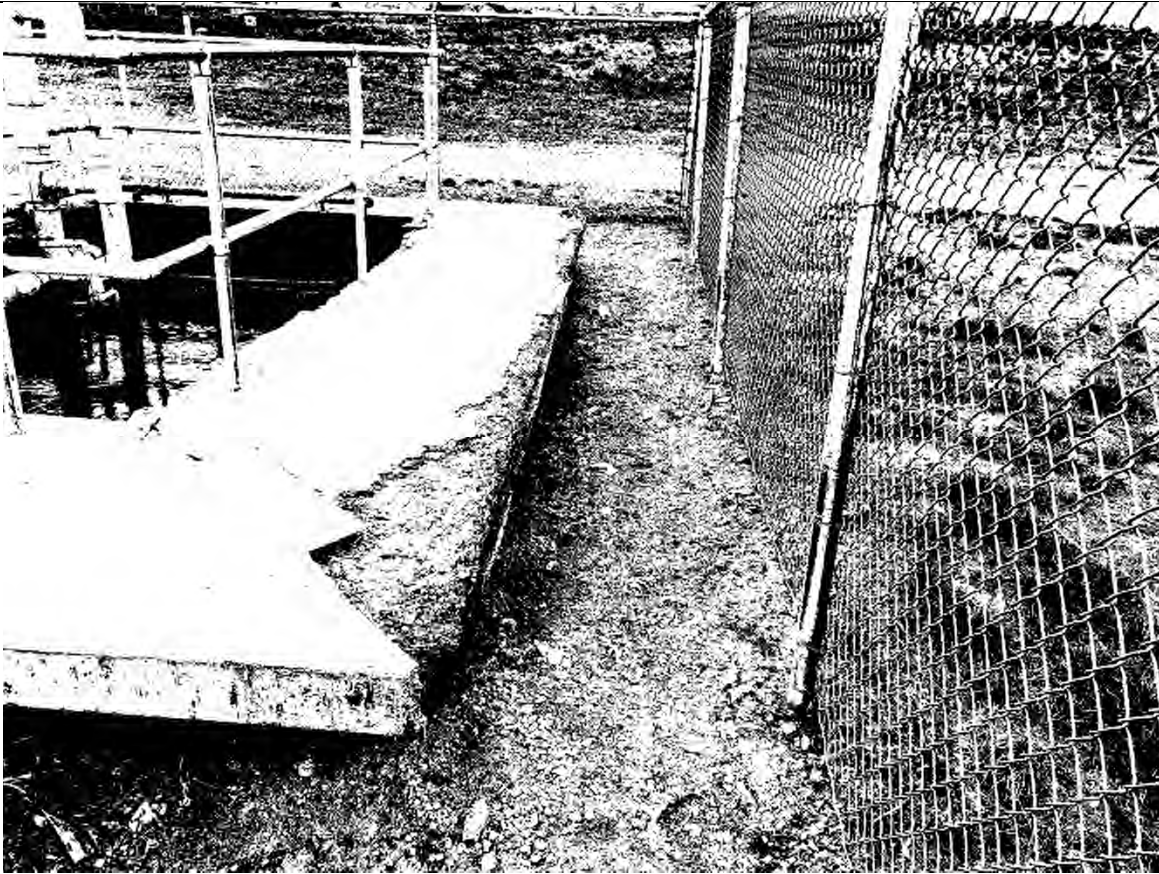
Photo 7 (4/15/2019) – Existing concrete cantilever walkway along north side of plant. Photo shows that concrete deterioration has increased since previous years with additional rebar exposure.
