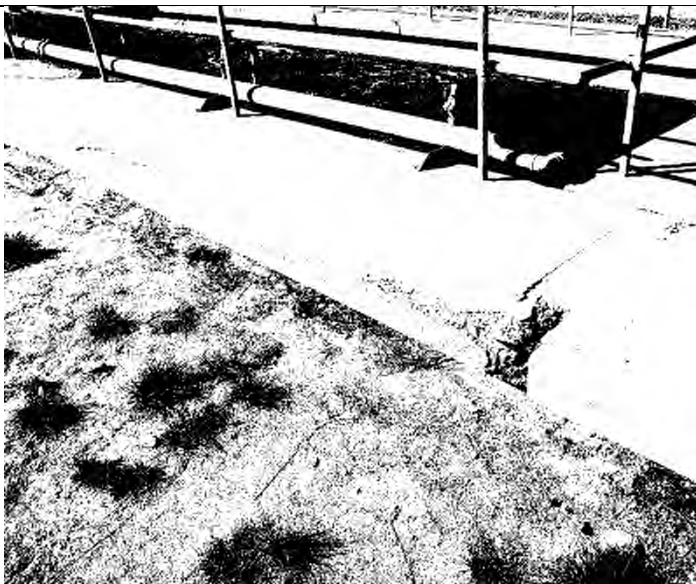
Photo 2 (9/13/2017) – Existing concrete cantilever walkway along east side of plant. Photo shows concrete cracks, spalling, and exposed aggregate.
