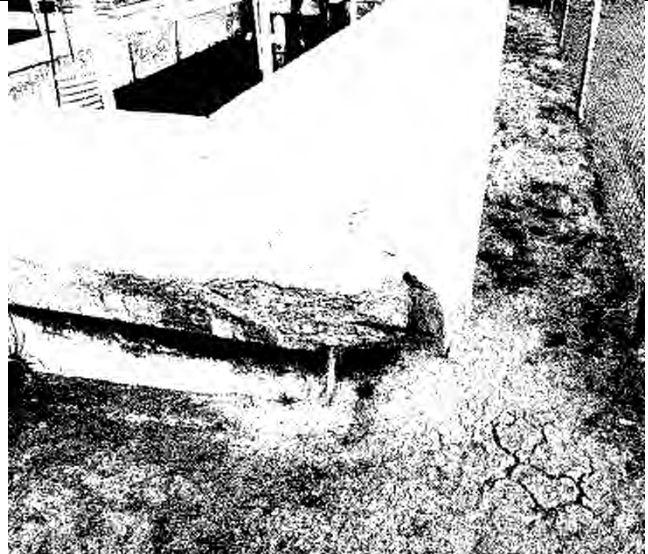
Photo 9 (4/15/2019) – Existing concrete cantilever walkway at southwest corner of plant. Some additional deterioration has occurred since 2018 as evidenced by aggregate collecting on the ground (see Photo 6).
